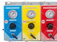
Gas Distribution Panel
